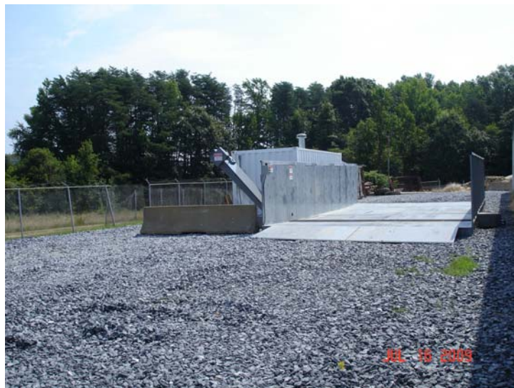
Marine Corps, (CIBRF) 18' x 35' pad with conveyor (left side). Drive thru configuration Filtration equipment and pressure washer installed in all-weather enclosure Rack installed on slightly improved surface
