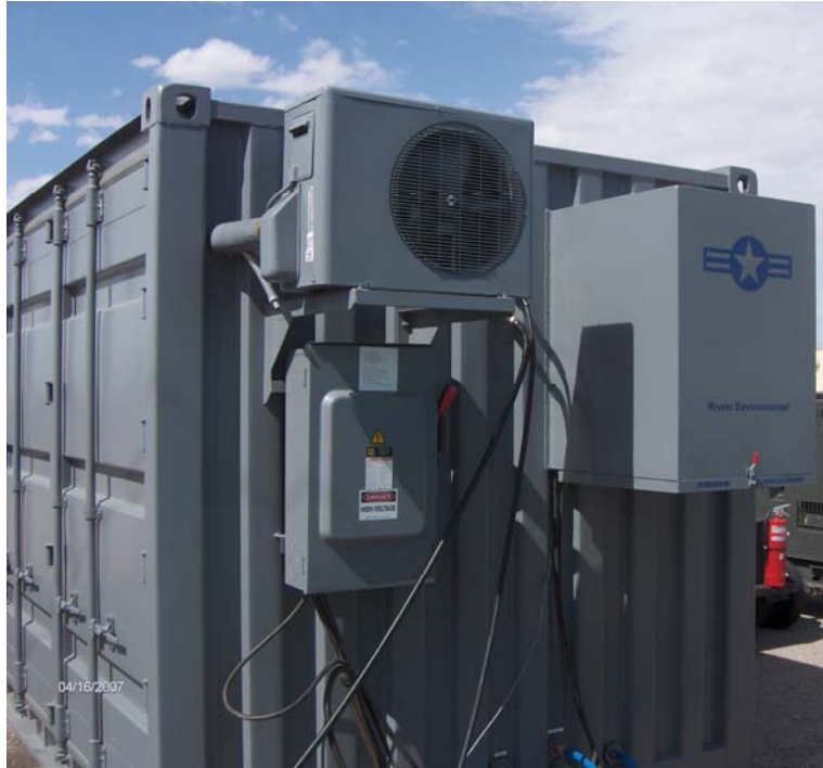
Hardened Wash Bay enclosure with air conditioning, heat and custom desert air filter, painted Air Force grey
