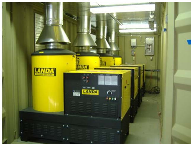
4 hot water pressure washers in hardened enclosure
