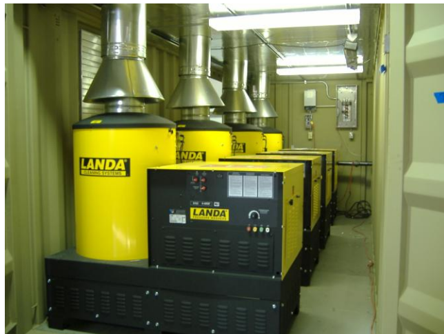
4 hot water pressure washers in hardened enclosure
