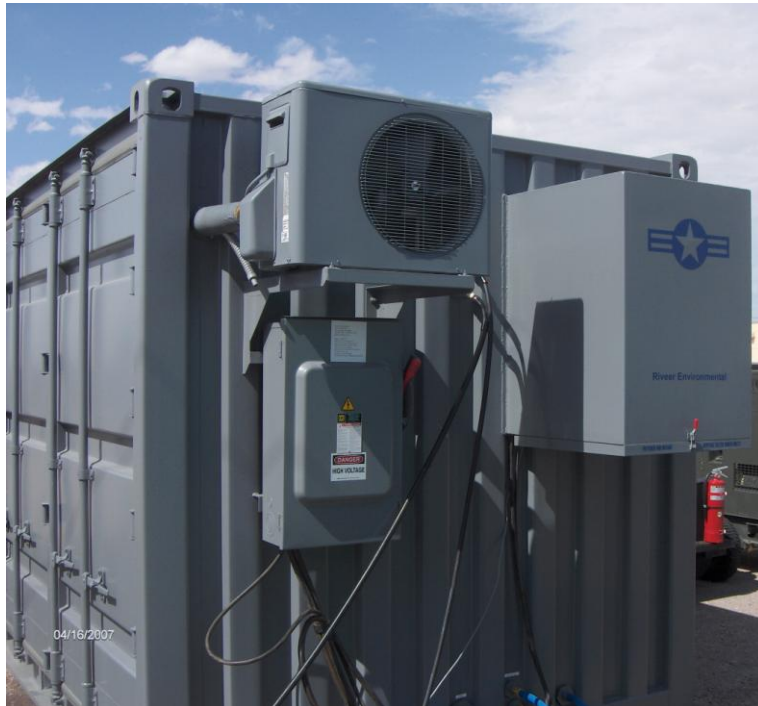
Hardened Wash Bay enclosure with air conditioning, heat and custom desert air filter, painted Air Force grey
